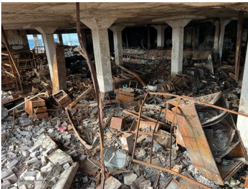
Photograph 7: Showing the extensive fire damages looking throughout the second floor of the building.
