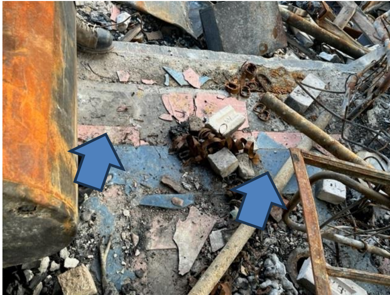
Photograph 3: Showing an example of the asbestos blue and red vinyl floor tiles located at the Site.
