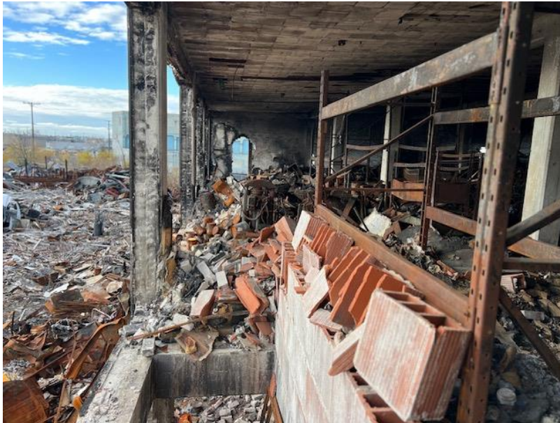
Photograph 6: Showing an example of the non-asbestos brick mortar located at the Site.
