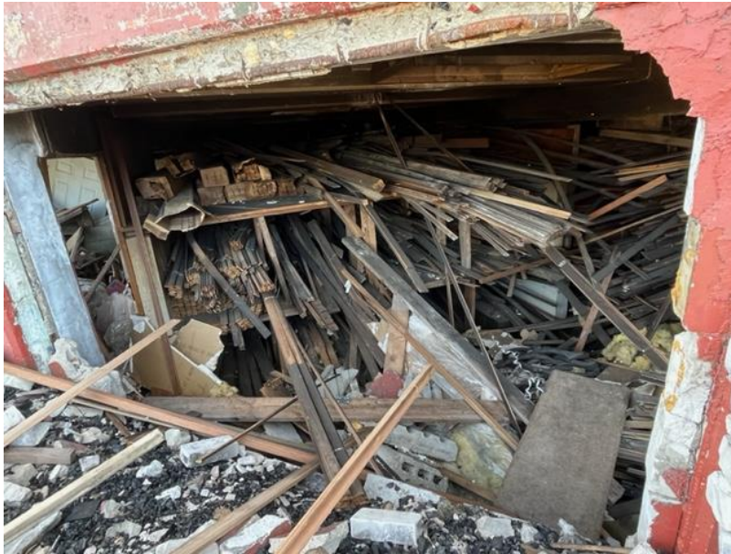
Photograph 10: Showing the extensive fire damages in the basement of the building which has no access at the time of assessment.
