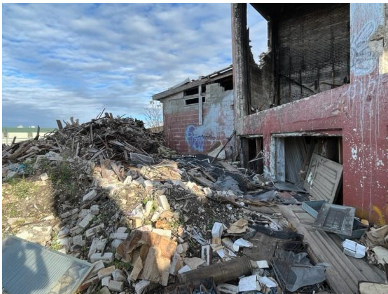
Photograph 11: Showing the extensive fire damages within the exterior of the building.
