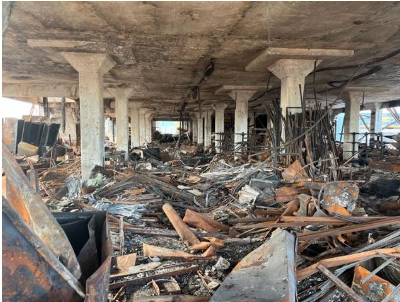
Photograph 8: Showing the extensive fire damages looking throughout the main floor of the building.
