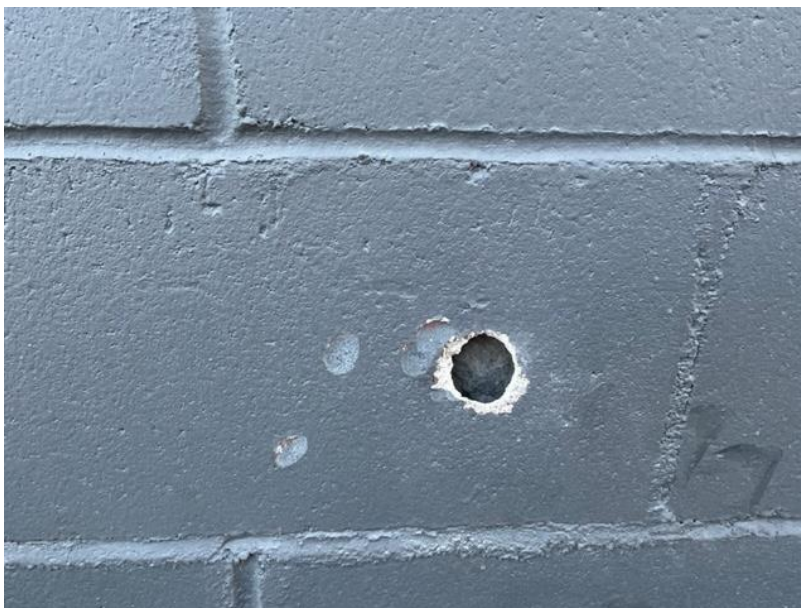
Photograph 9: Showing a hole in the cinder block exterior wall observing to have no vermiculite within the walls.
