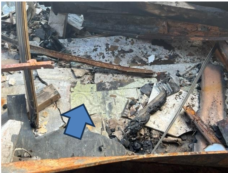
Photograph 2: Showing an example of the asbestos white vinyl floor tiles located at the Site.
